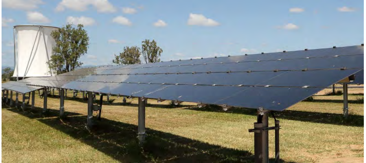
Figure 4-1 First Solar modules and a single axis tracker installed at the Gatton Research Facility in Queensland.
