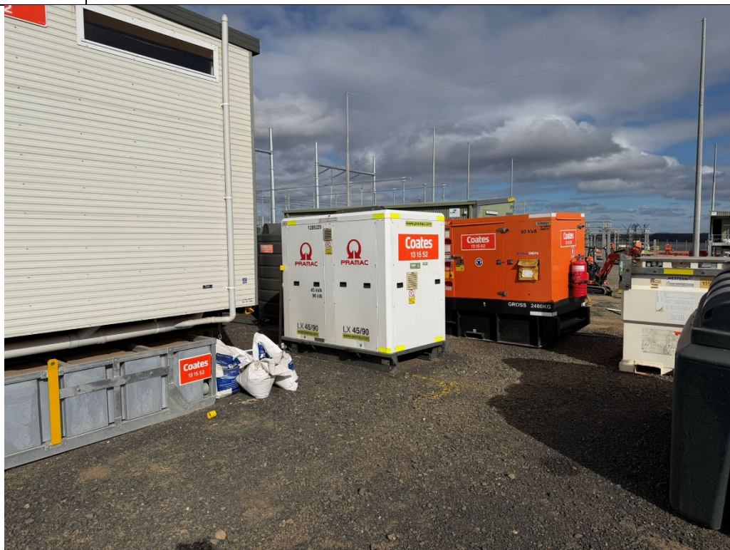
Photo 9 Transgrid / Enerven compound, showing diesel generator and AST.
