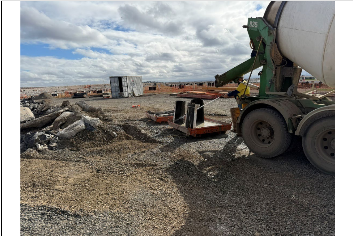
Photo 10 Transgrid / Enerven worksite, showing concrete washout using trays rather than a dedicated double-lined pit.
