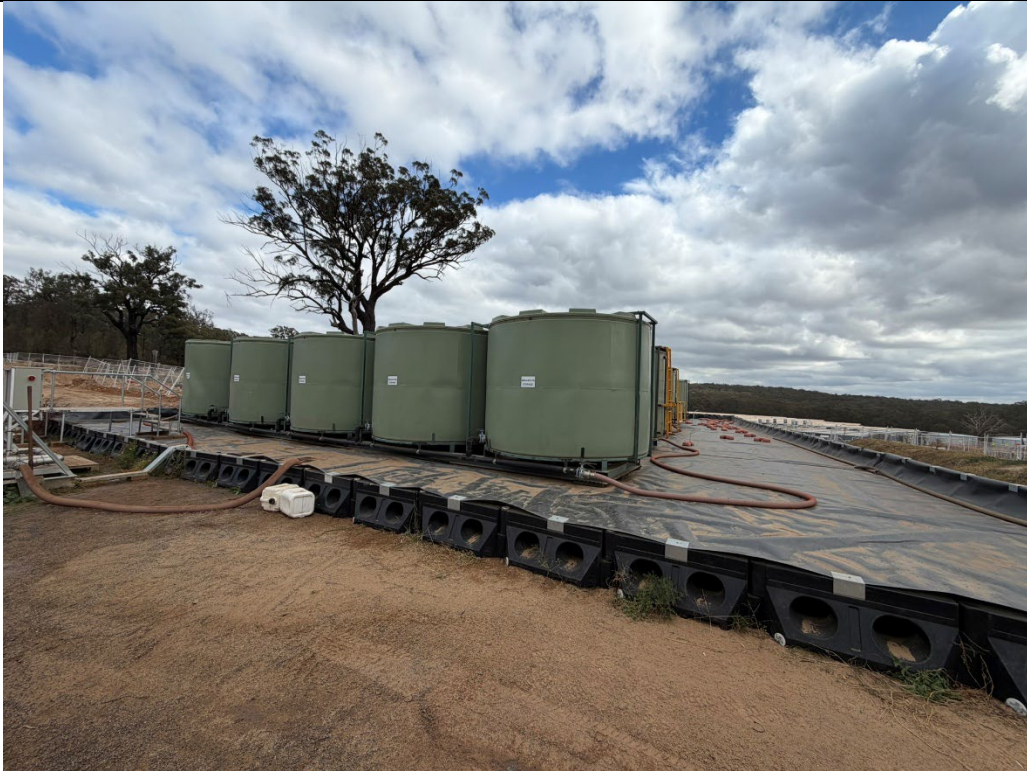
Photo 14 Wastewater treatment plant adjacent to workers camp.
