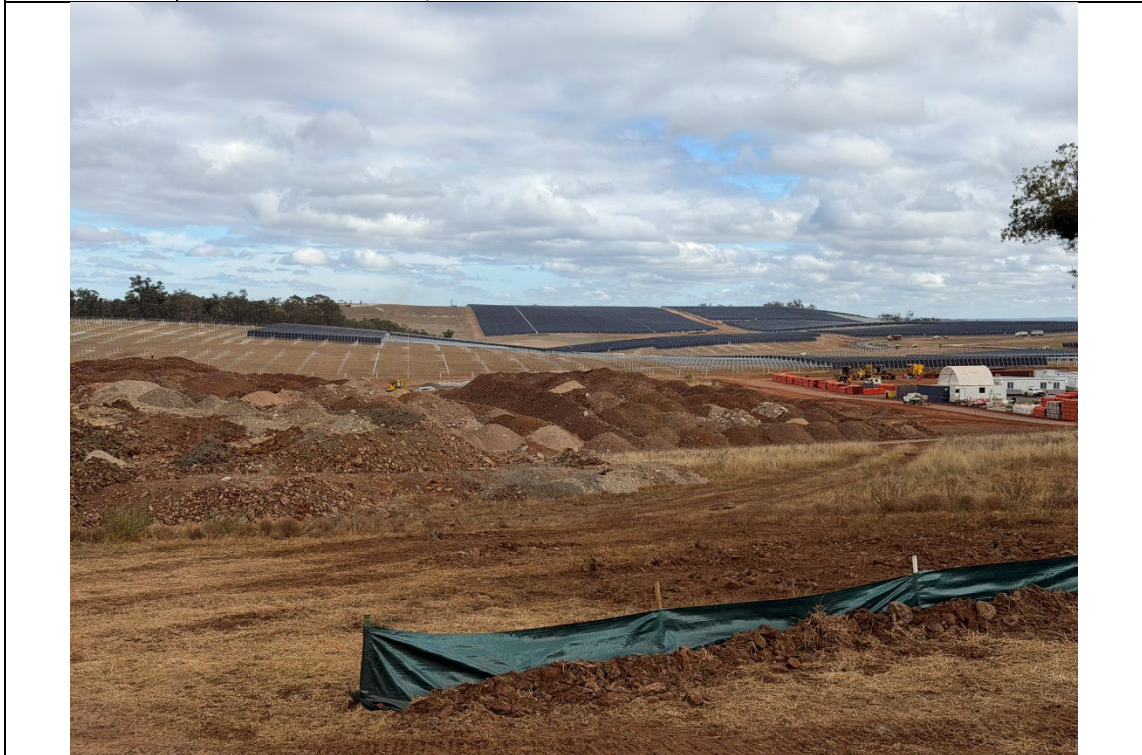
Photo 11 View from Transgrid / Enerven worksite, showing non-conforming stockpiles awaiting rock screening.
