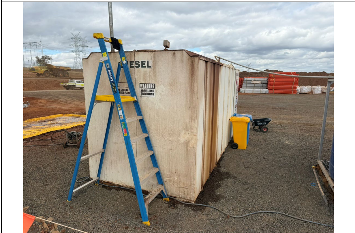
Photo 17 Diesel AST at DTI subcontractor site, showing evidence of leaks to surrounding gravel hardstand.
