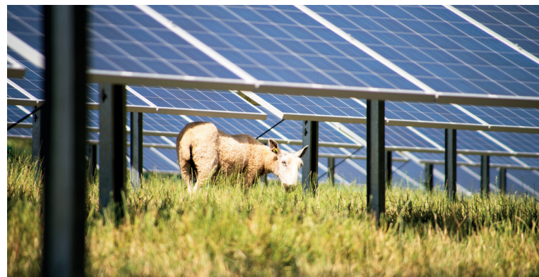
• Parque Solar Marley Thatch, Lightsource bp, Inglaterra
